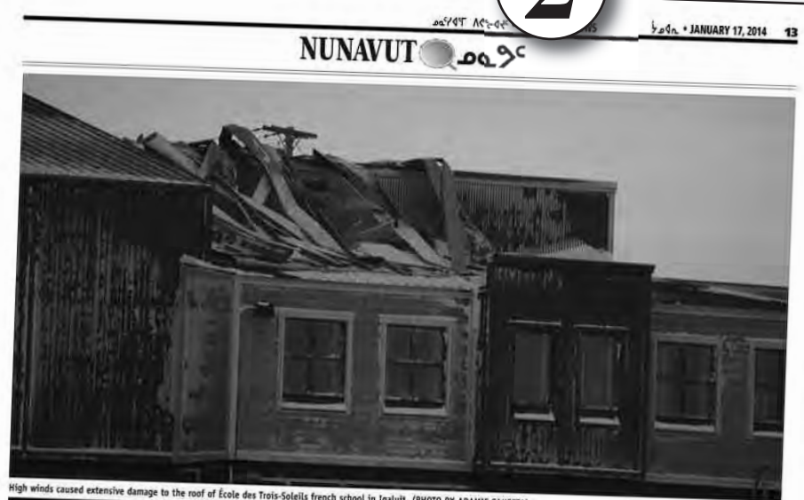
High winds caused extensive damage to the roof of École des Trois-Soleils french school in Iqaluit. (PHOTO BY ADAMIE SAKKEETA)
